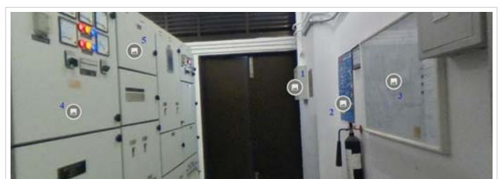
Figure 2: Screenshot of VR Training view within switch-room.
